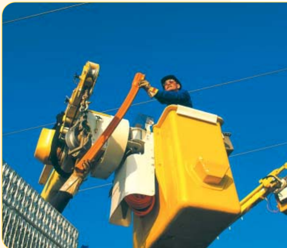
Maritime Electric serves approximately 67,000 customers on Prince Edward Island.
