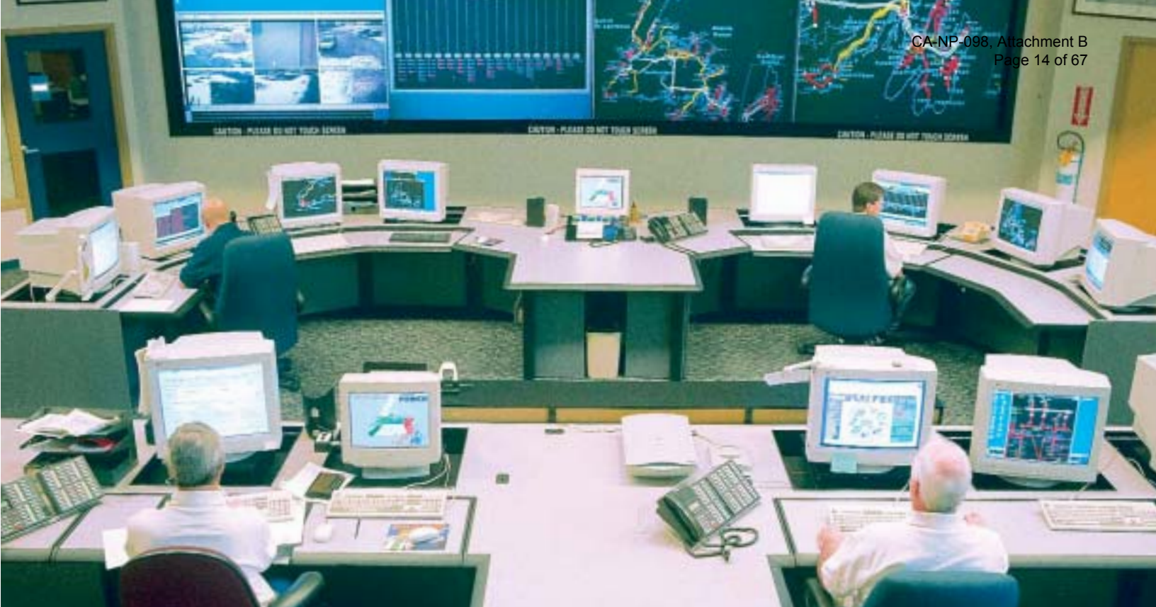
Newfoundland Power's investment in state-of-the-art System Control and Data Acquisition technologies enables the Company to remotely control more of its electrical system than ever before.
