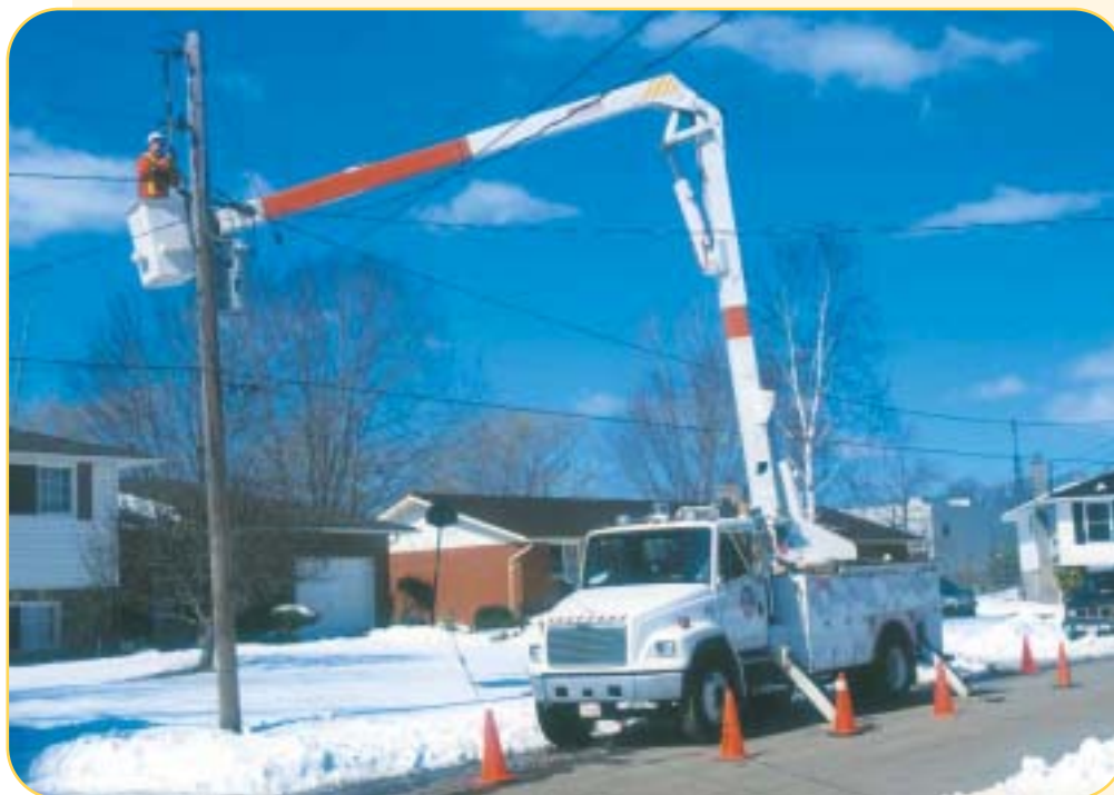
Canadian Niagara Power serves 15,000 customers in the Town of Fort Erie, Ontario.
