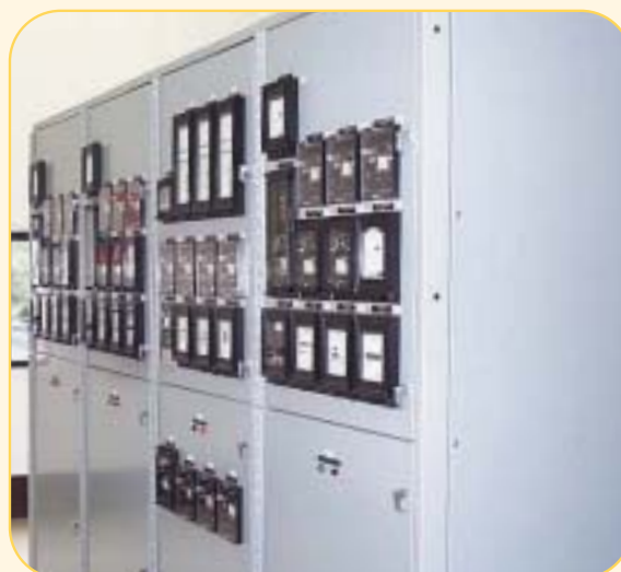
Control panel for Mollejon's three turbine generators
